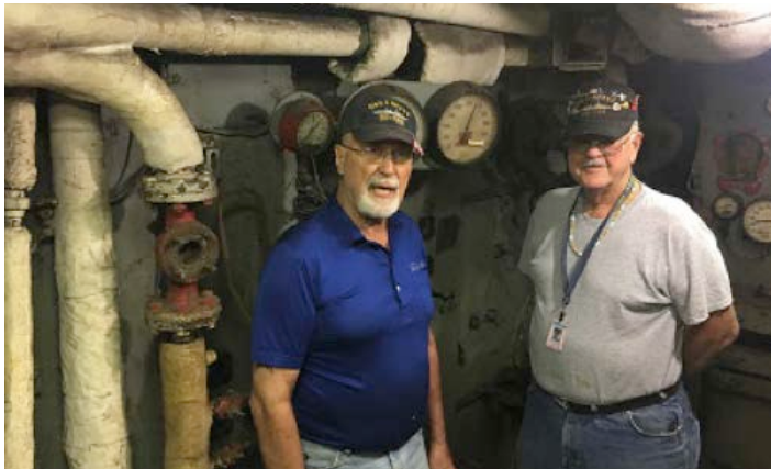
Boiler Tender John Hudak and Boatswain Ken McCullough in After Fire Room. Good to visit the snipes. John has great plans for opening the Fire-Room to visitors.
