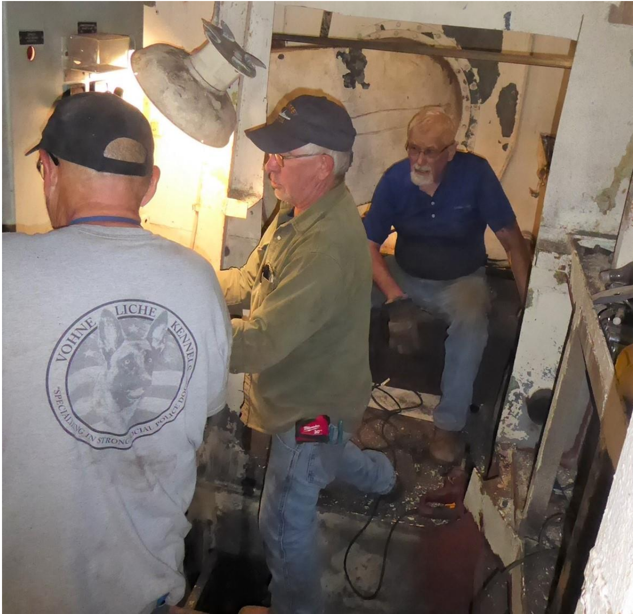
Well Done Ernie Doyle, Harry Stoner, and John Hudak Opening Aft Engine Room into the Aft Fire Room during Mini-Workparty 24-30 September with Mike Honsinger
